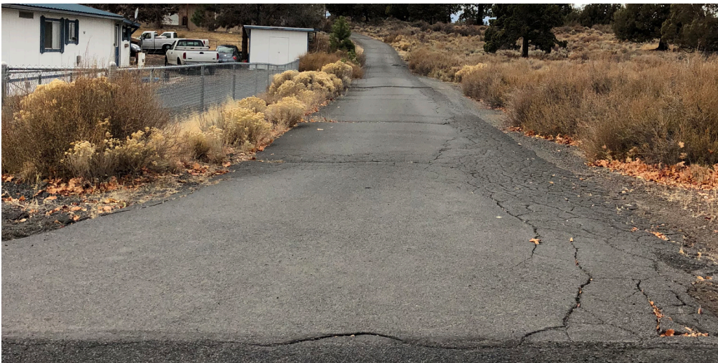
Pavement conditions on Raintree Court
